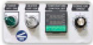
Tunnel Control Panel
