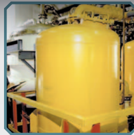
Equipment and Tanks
