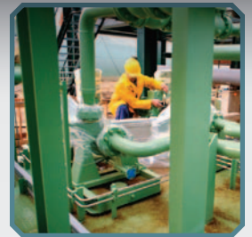
Pipes and more
